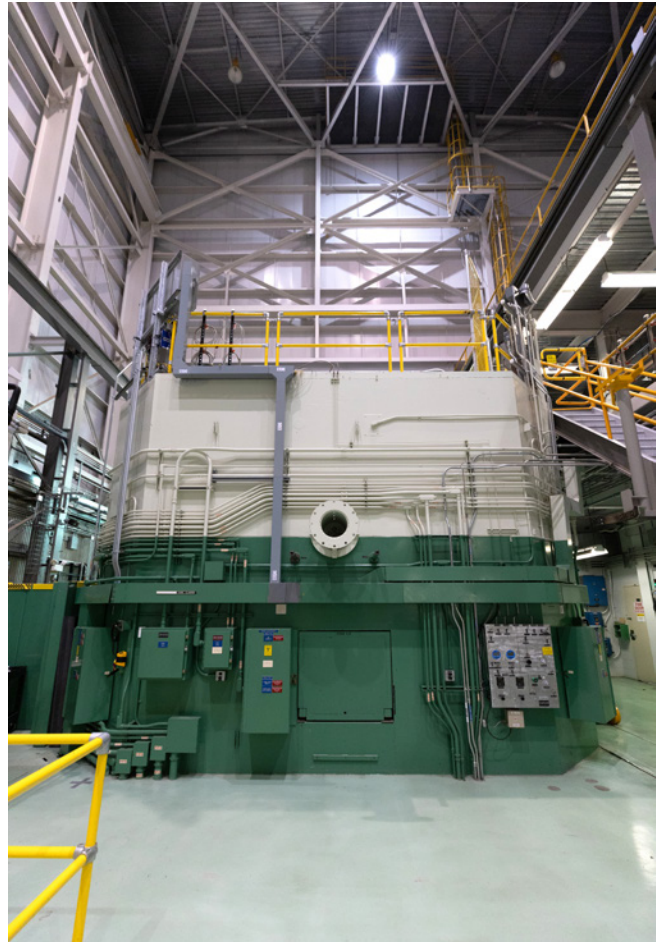
Researchers at INL's TREAT reactor evaluate the performance of fuels and structural materials, aiding the development and commercialization of new technologies.
